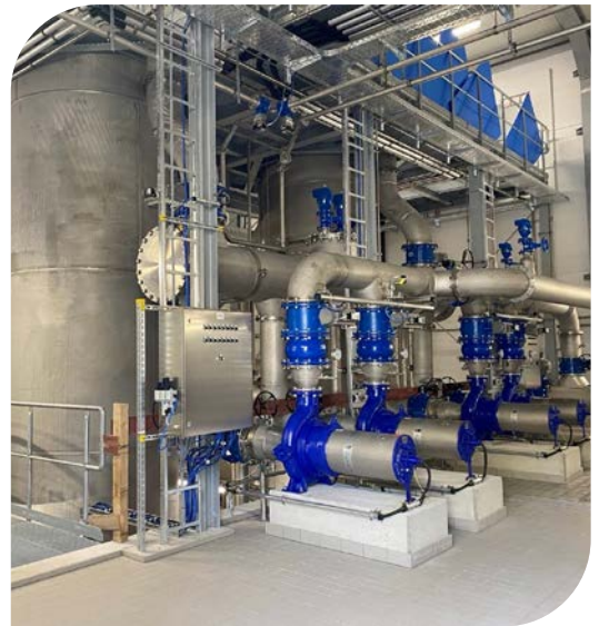
Fig. 2: The new SEC system at the Osthofen Water Treatment Plant for softening drinking water
